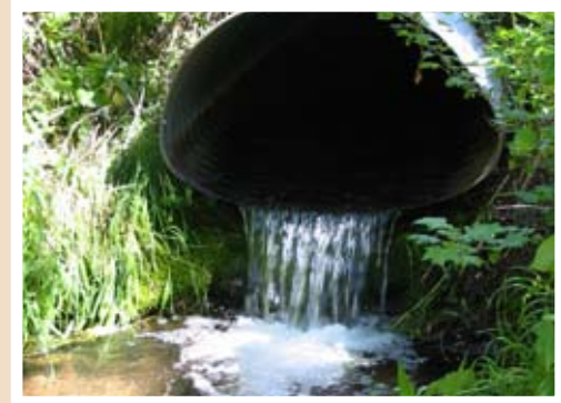
Highway culvert impassable to fish by Matt Blank
